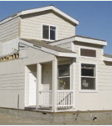
Using a crane, the top module was placed over the ground floor. Note the details of the inter-floor connection and of the foundation wall.
